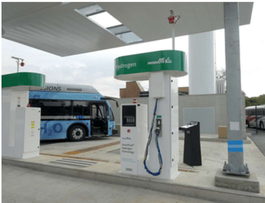
SARTA Hydrogen Fuel Cell Bus Refueling Station Canton, Ohio
