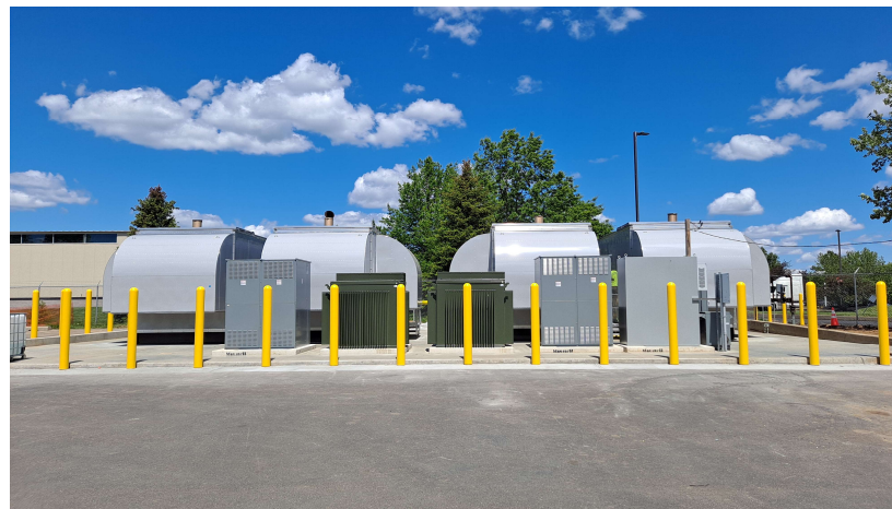
Peaking Generation – Retail Distribution Center - PA
