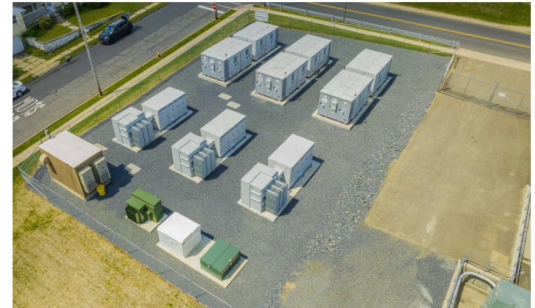
Battery Project – South River, NJ
