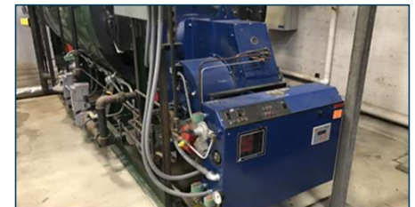
BOILER BURNER AT THE COURTHOUSE
