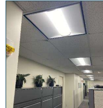
LED FIXTURES AT ADMINISTRATION BUILDING
