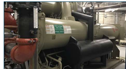
CHILLER AT THE JUSTICE CENTER
