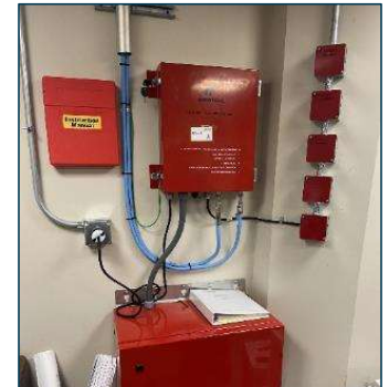
FIRE ALARM SYSTEM AT PORTUNE CENTER
