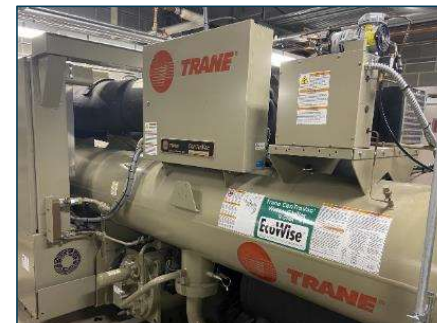
CHILLER AT JUVENILE DETENTION CENTER
