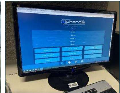
LIGHTING CONTROL SYSTEM AT COURTHOUSE
