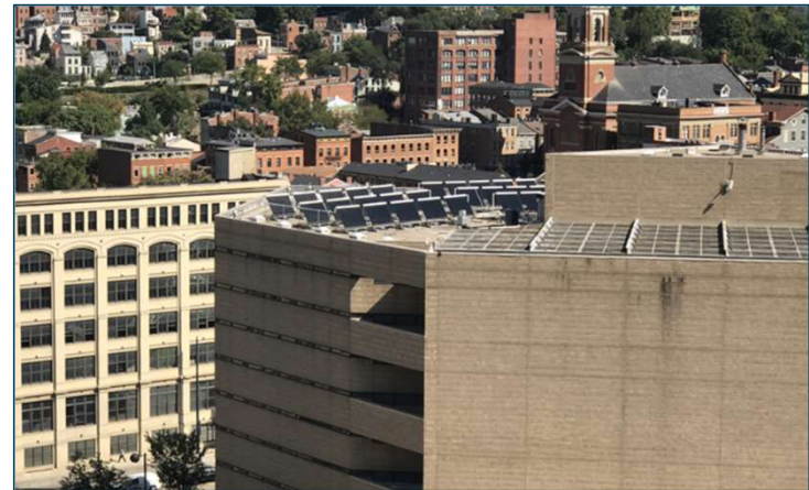
SOLAR THERMAL PANELS AT THE JUSTICE CENTER
